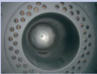
Internal view of combustion chamber
